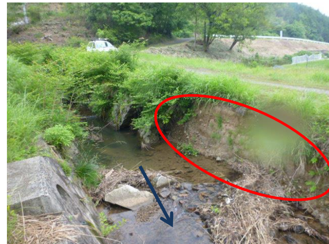
左岸石積み護岸の崩れ
